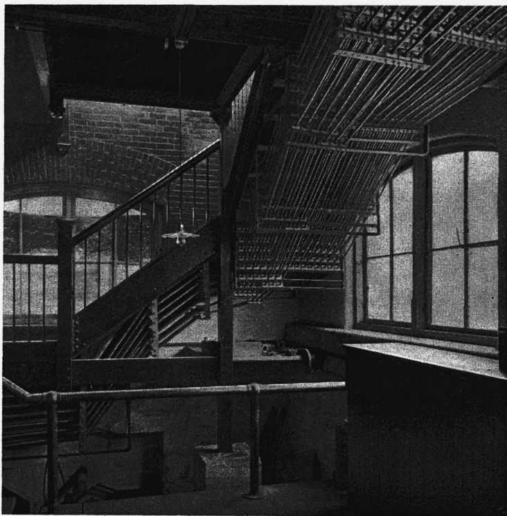
FIG. 8. LARGE GROUP OF WIRES, WELL SUPPORTED.
